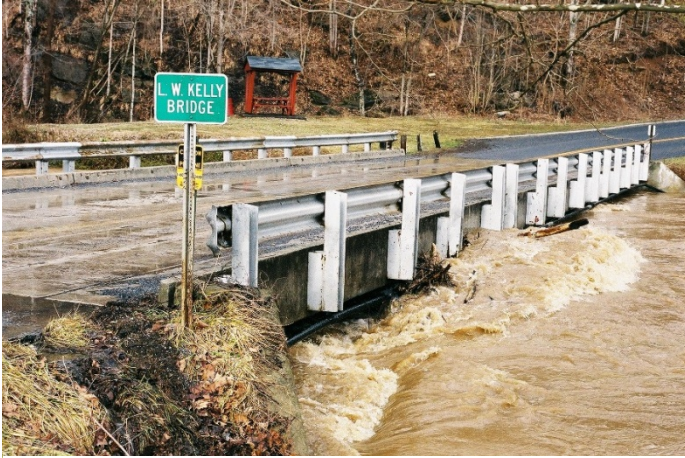
View of flooding at Baughman Street Bridge in Marion. The bridge itself becomes a barrier during times of high water.
