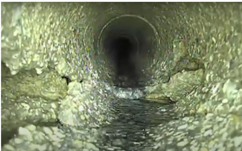
Figure 3.4.1 – Deteriorated Section of Concrete Sewer Line
