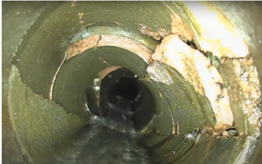
Figure 3.4.2 – Collapsed Section of Terracotta Sewer Line
